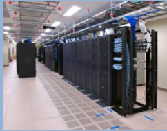
Data Centre Planning and Relocation
